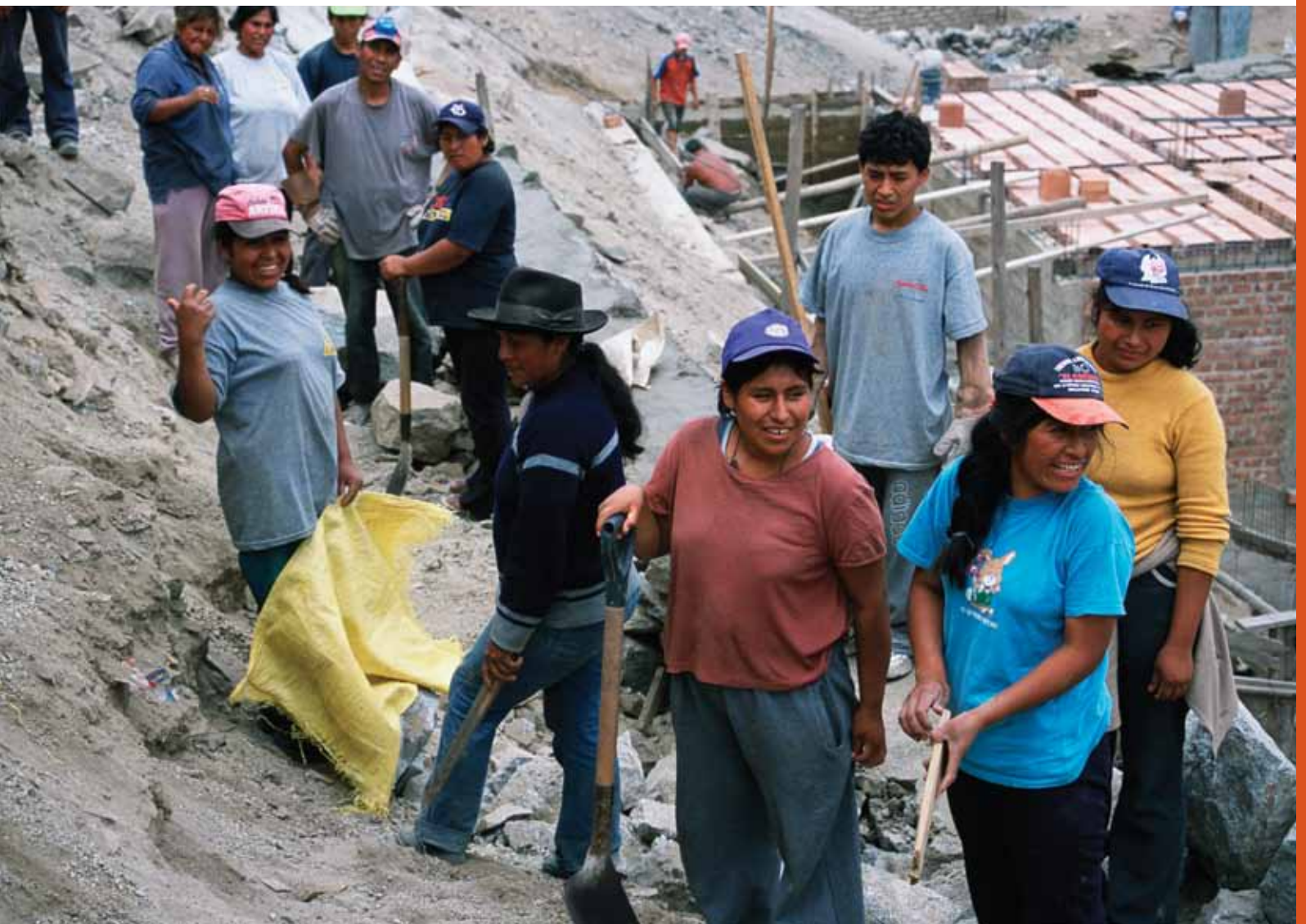
Residents of Amauta-B shantytown in Peru work to build a retaining wall in their community.
